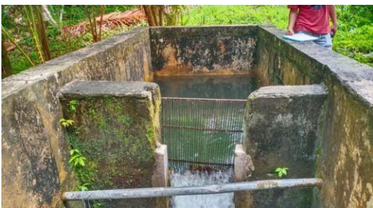
Gambar 6. Saringan ( Trash Rack )
